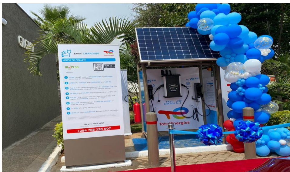
Figure 1: Photo depicting a solar EV charger commissioned in Total Energies Gigiri by Knight Energy a good example of collaboration between different parties
